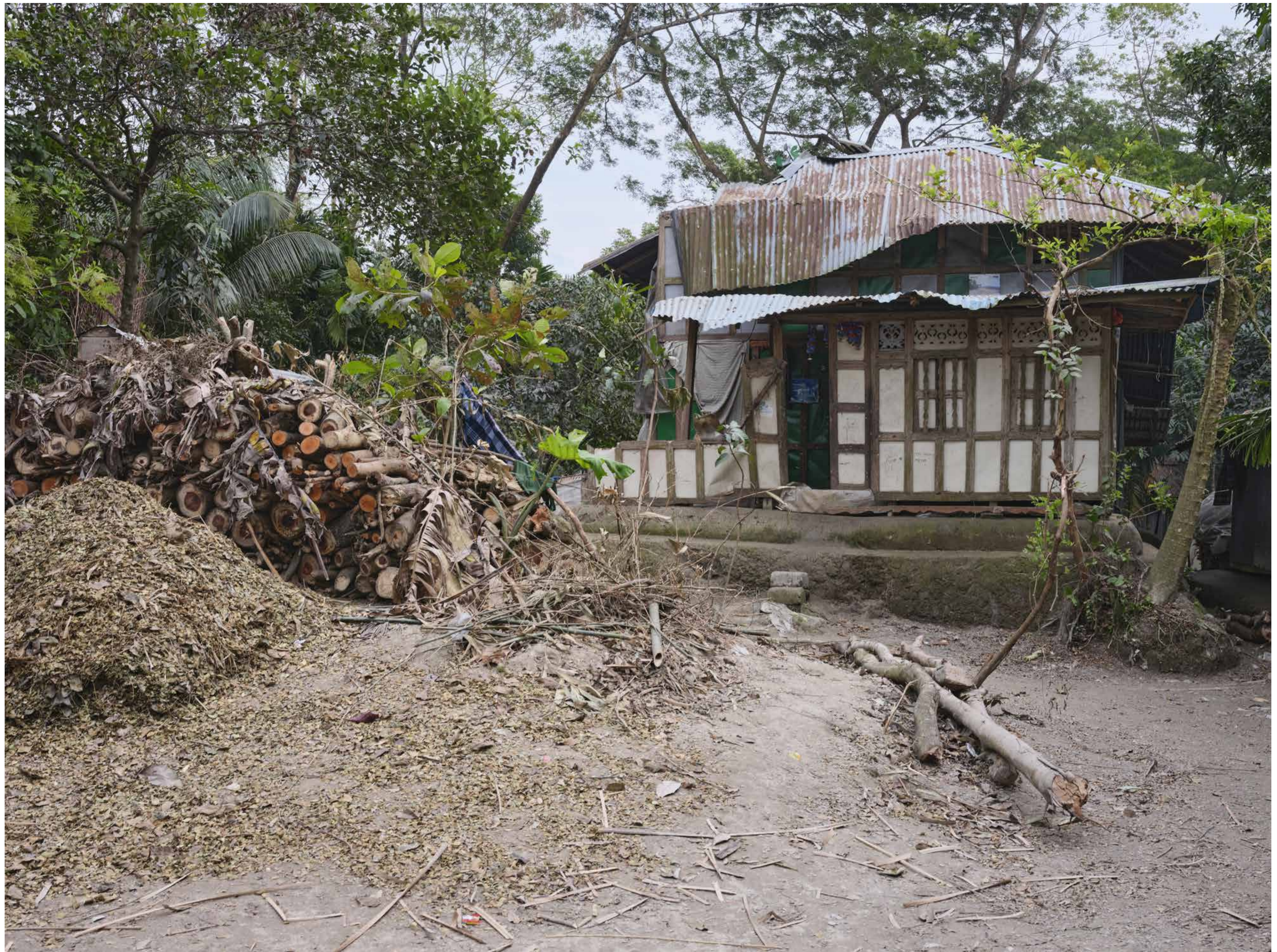
Tin roof of a home damaged by the Cyclone Bulbul, Mehendiganj Upazila, Barisal District, Barisal Division.
