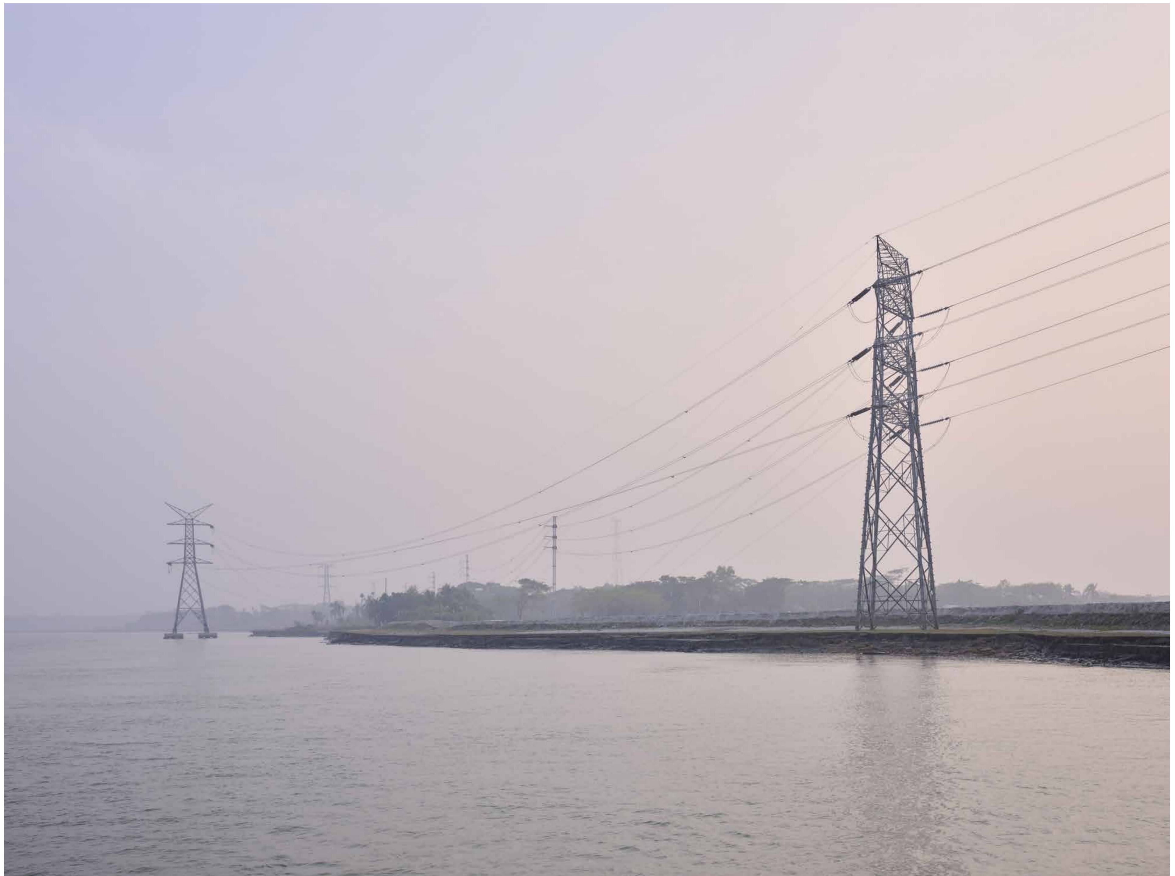
Electricity pylons damaged by river erosion. Meghna River, Barisal Division.
