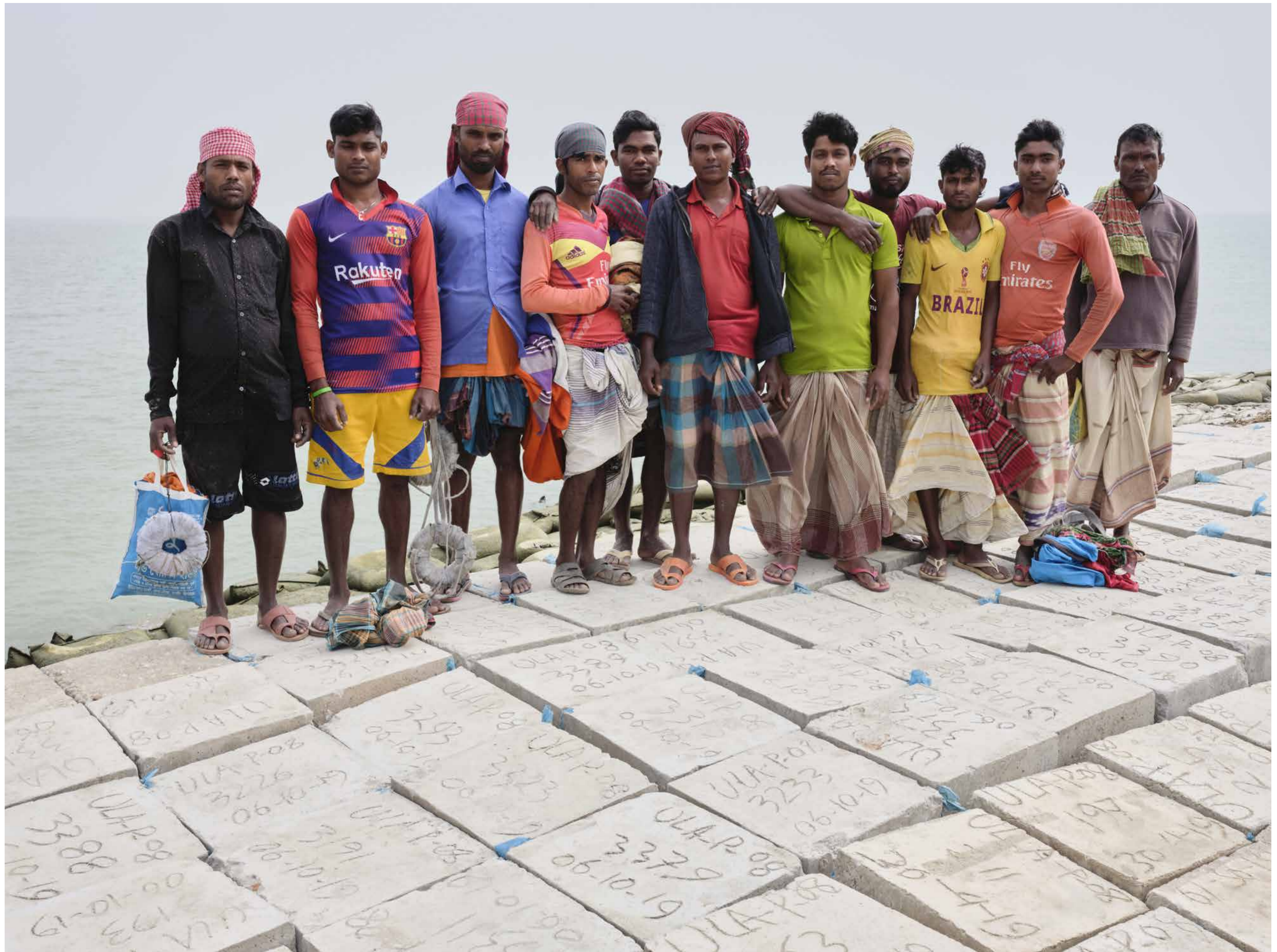
Municipality workers installing concrete blocks to strengthen the riverbank. Ulania, Mehendiganj Upazila, Barisal District, Barisal Division.
