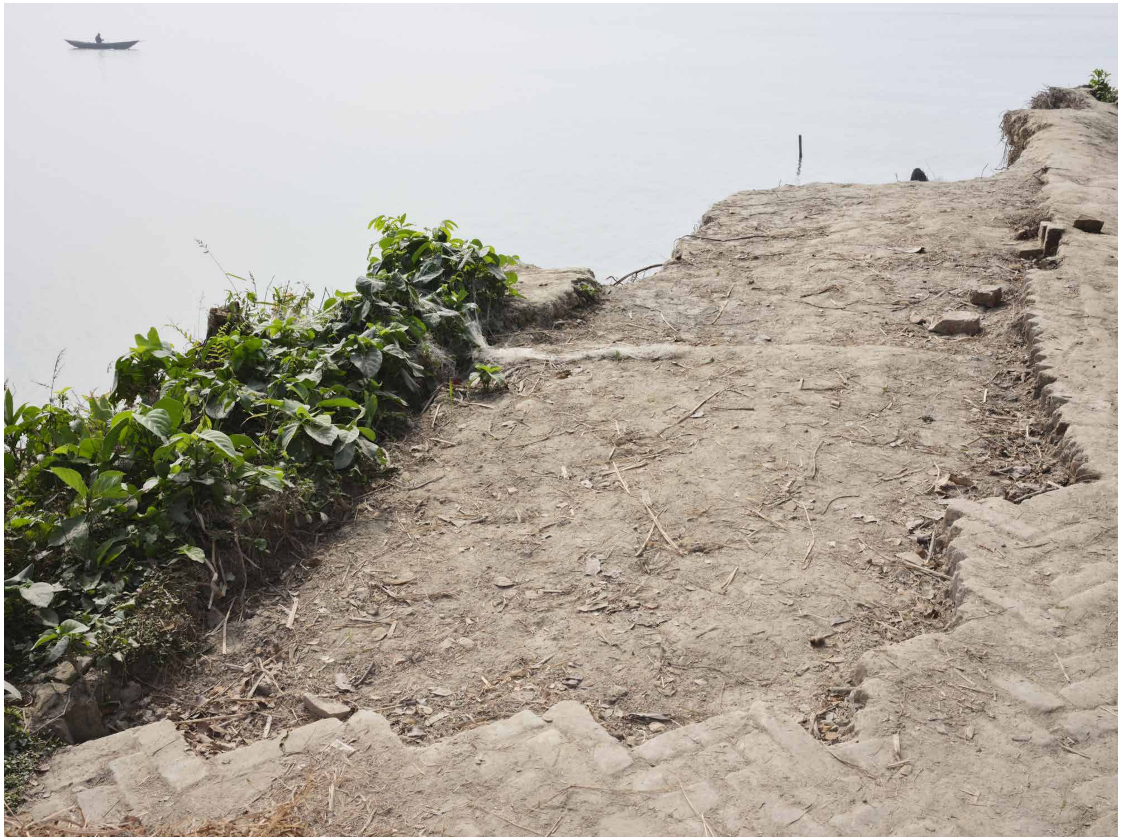
Country road swallowed by river erosion. Char Hogla, Mehendiganj Upazila, Barisal District, Barisal Division.
